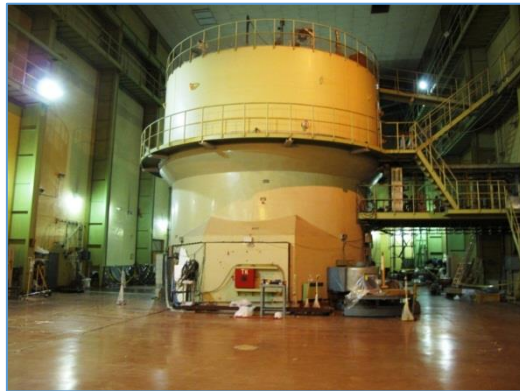
Figure 2. Research reactor RA
